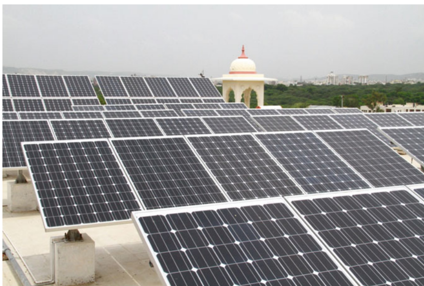
Fig. 4.48 Roof-mounted SPV panels, Aranya Bhawan (© Tapan Kumar Ghoshal)
