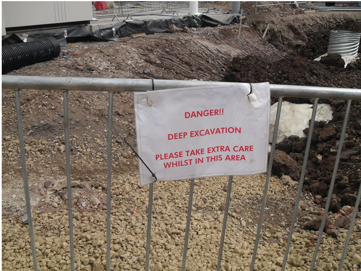
Figure 5.2 Danger – Deep Excavation
